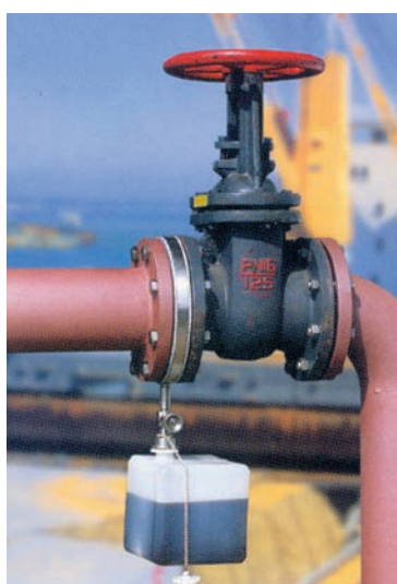
In-line drip sampler for fuel oil with mounted sample container
